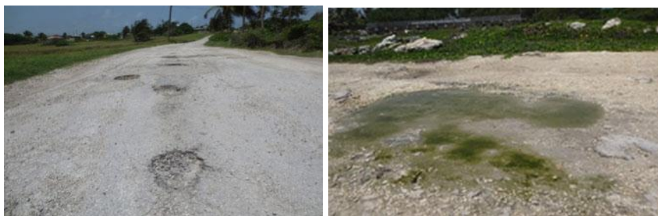
Figure G7. Public access road to the tourist attraction at Animal Flower Cave (left) and car park at the Animal Flower Cave (right), both in need of repairs.
